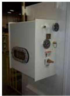
Figure 7. External visible break with gauges.
