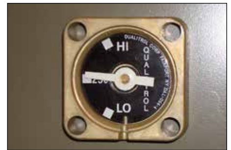
Figure 5. Liquid level gauge.
