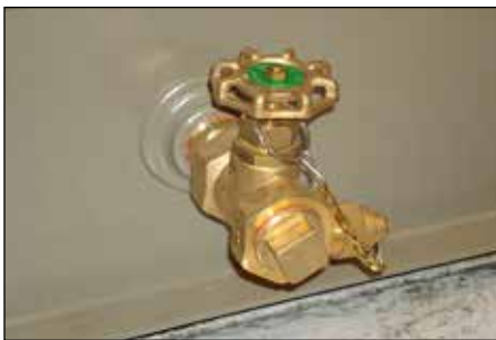
Figure 3. Drain valve with sampler.
